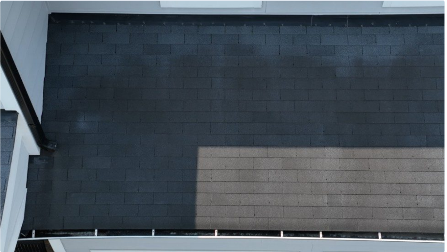
Fig. 6 — P3 — valley transition and gutter line. Localized surface discoloration recorded as a LOW observation.
