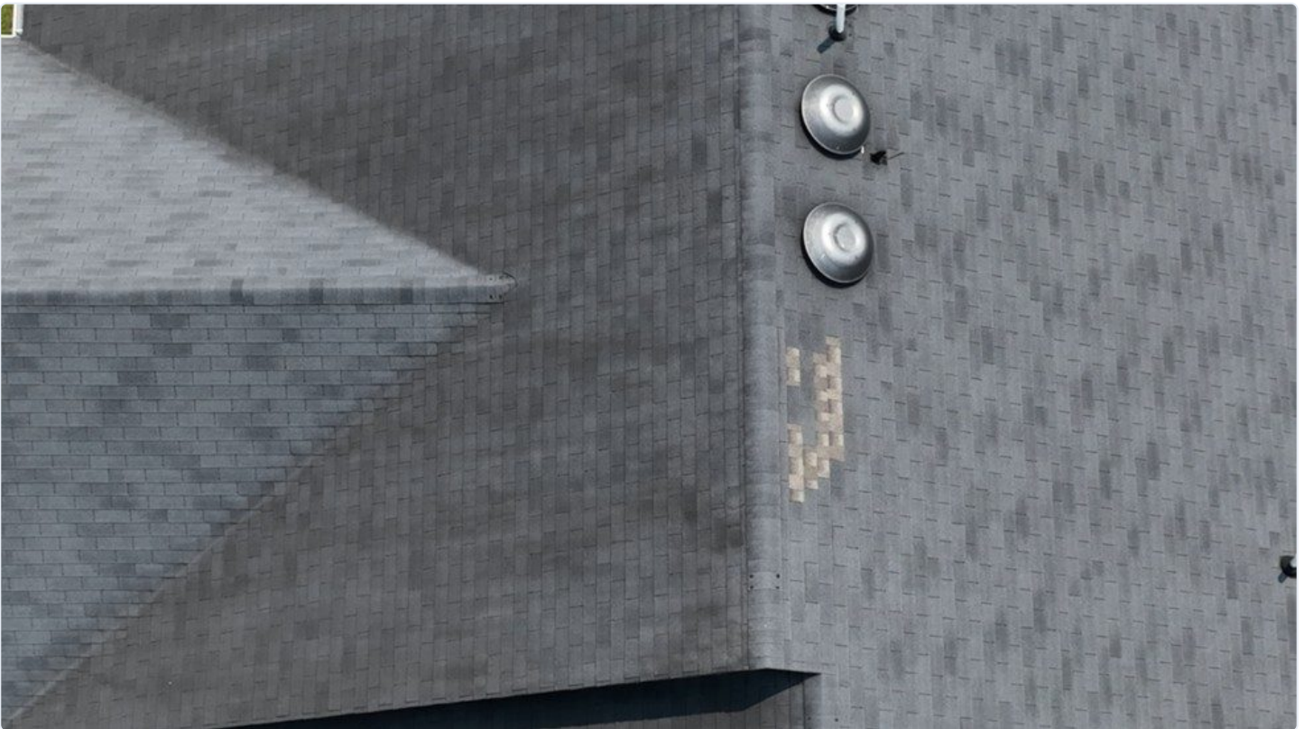
Fig. 4 — P1 — the same finding from the opposing approach. Two angles on one defect.
