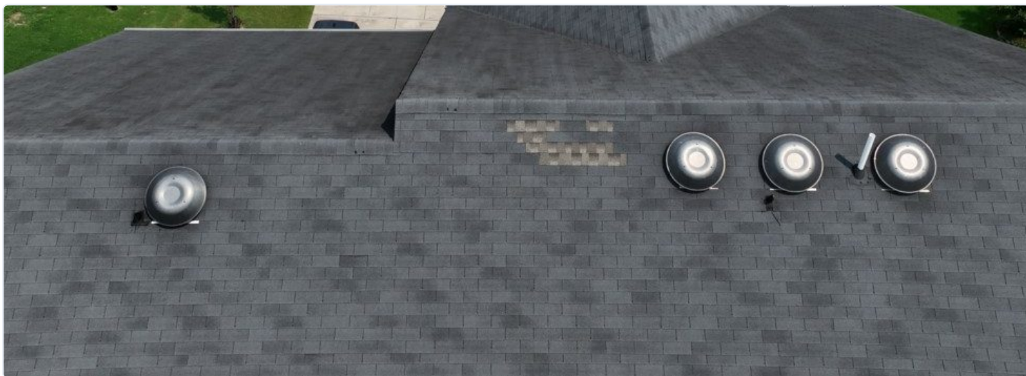
Fig. 2 — P1 front plane in context. Affected area sits immediately below the ridge; surrounding field, vents and ridge line intact.
