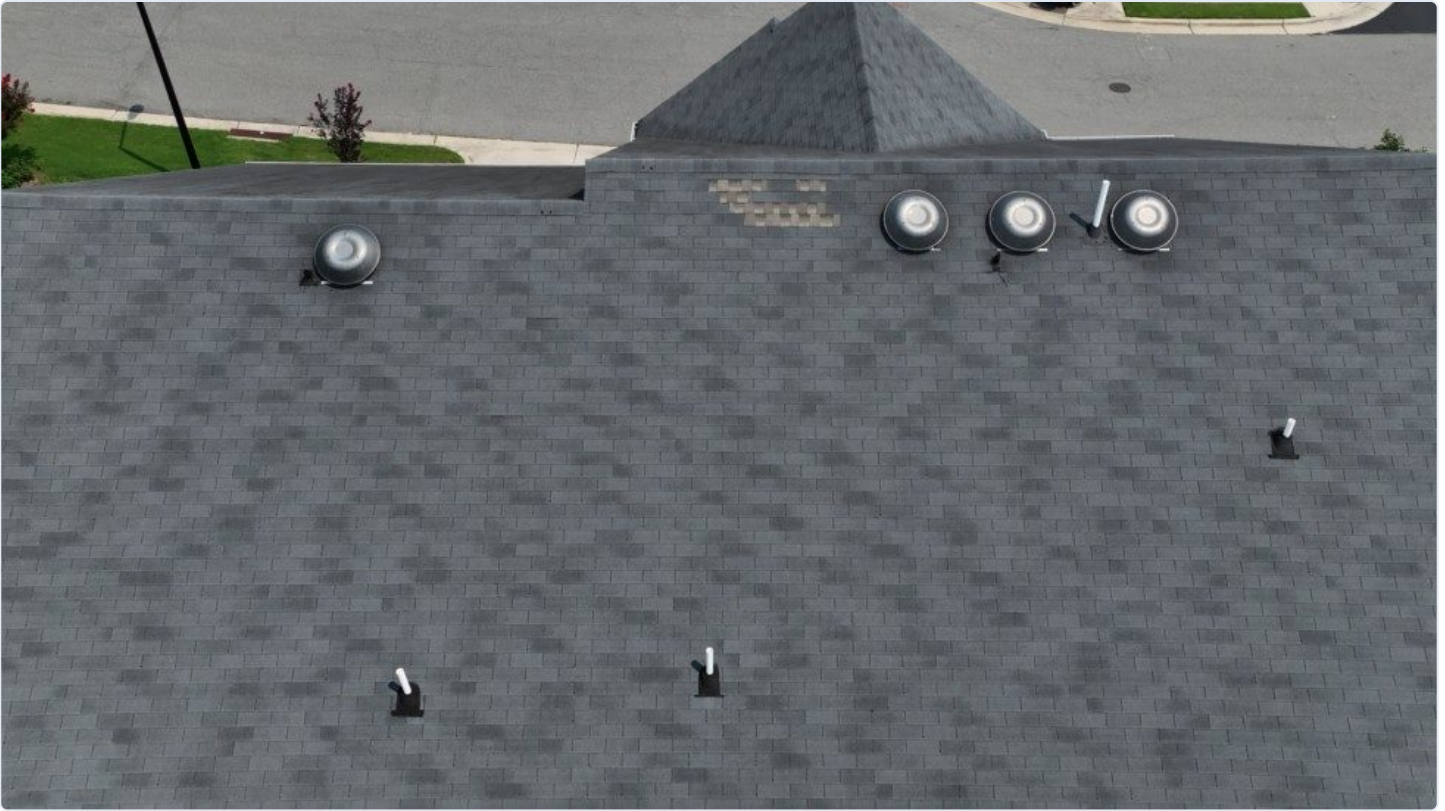
Fig. 3 — P1 — missing shingles along the upper ridge, underlayment exposed across the affected courses.
